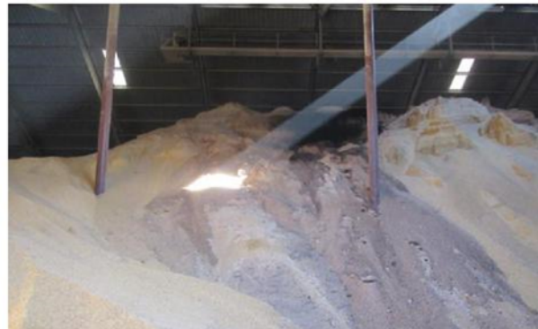
Interior support structures evaluated for heat or deformation from fire and unloading forces.
