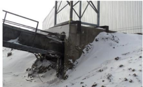
Close inspection for heat and fire damage to peripheral equipment, conveyors and support towers at vent points
