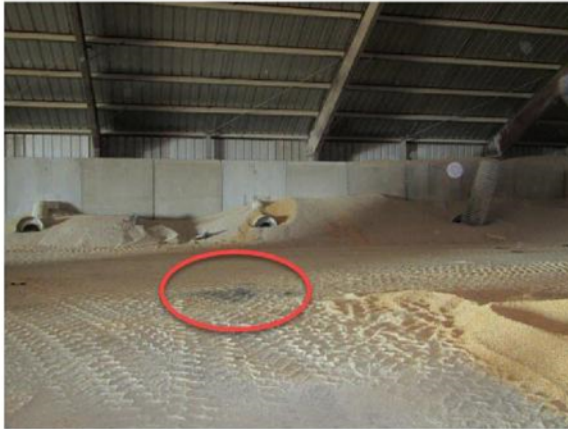
Older asphalt flat building floors may require close inspection from heavy equipment traffic
