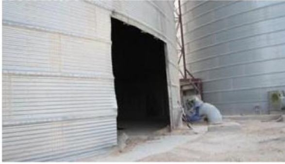
Access cut in bin side wall sheet to get at burning grain column
