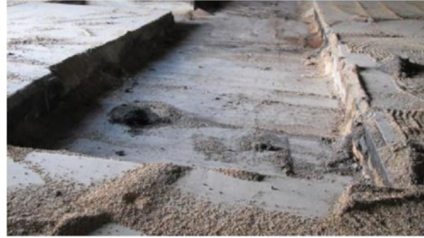
Air floor damage from heat, and process of removing grain.
