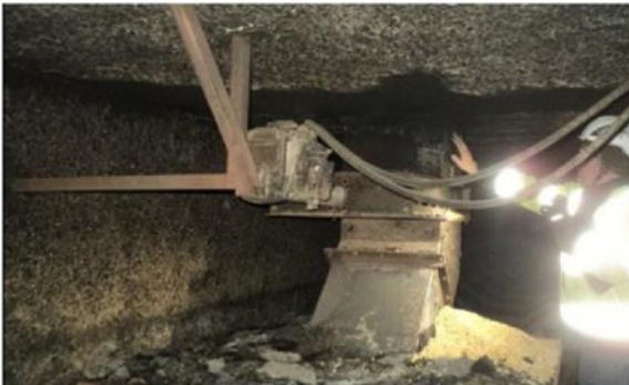
This concrete tunnel ceiling will need engineering and reclaim equipment replaced
